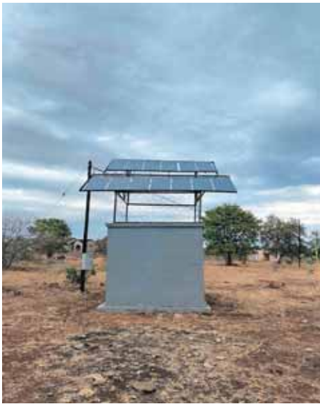
A solar-powered pump house at Mayephu Village.
