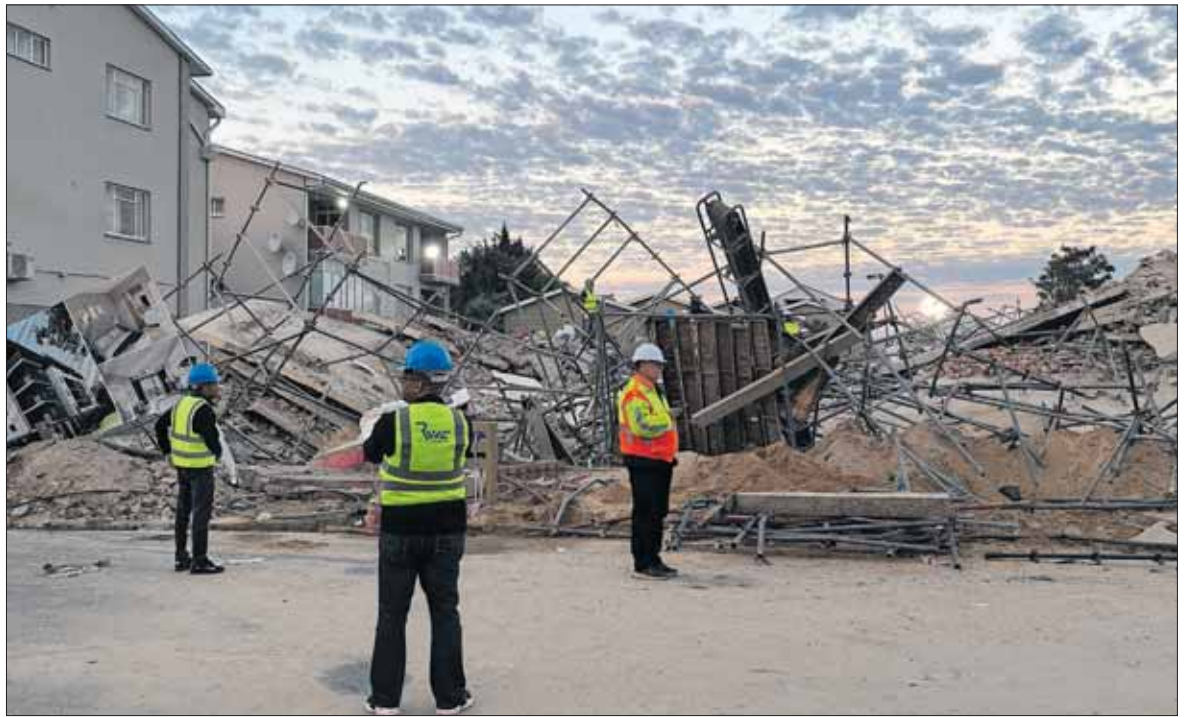
Tragedy: Officials at the building in George which collapsed on 6 May. Teams are still digging for the bodies of missing workers. Photo: Willie van Tonder/AFP
